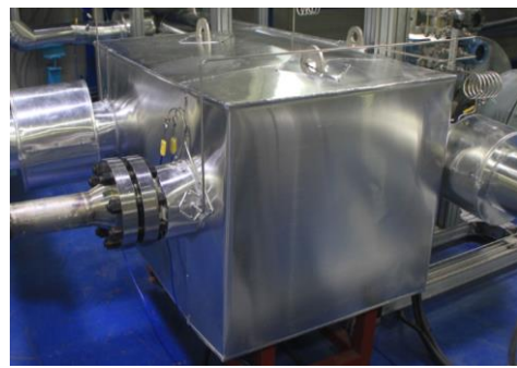
Fig. 2. The upgraded prototype helium circulator and the insulated recuperator installed in HeSS (2020)
